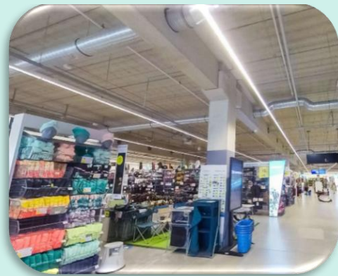
LEDs at Decathlon Unit Hofheim-Wallau, Germany
